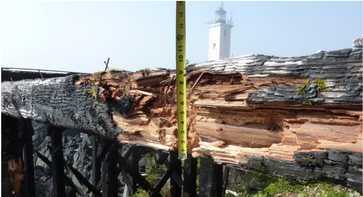
Figure 3. Wood material has lost integrity due to decay.
