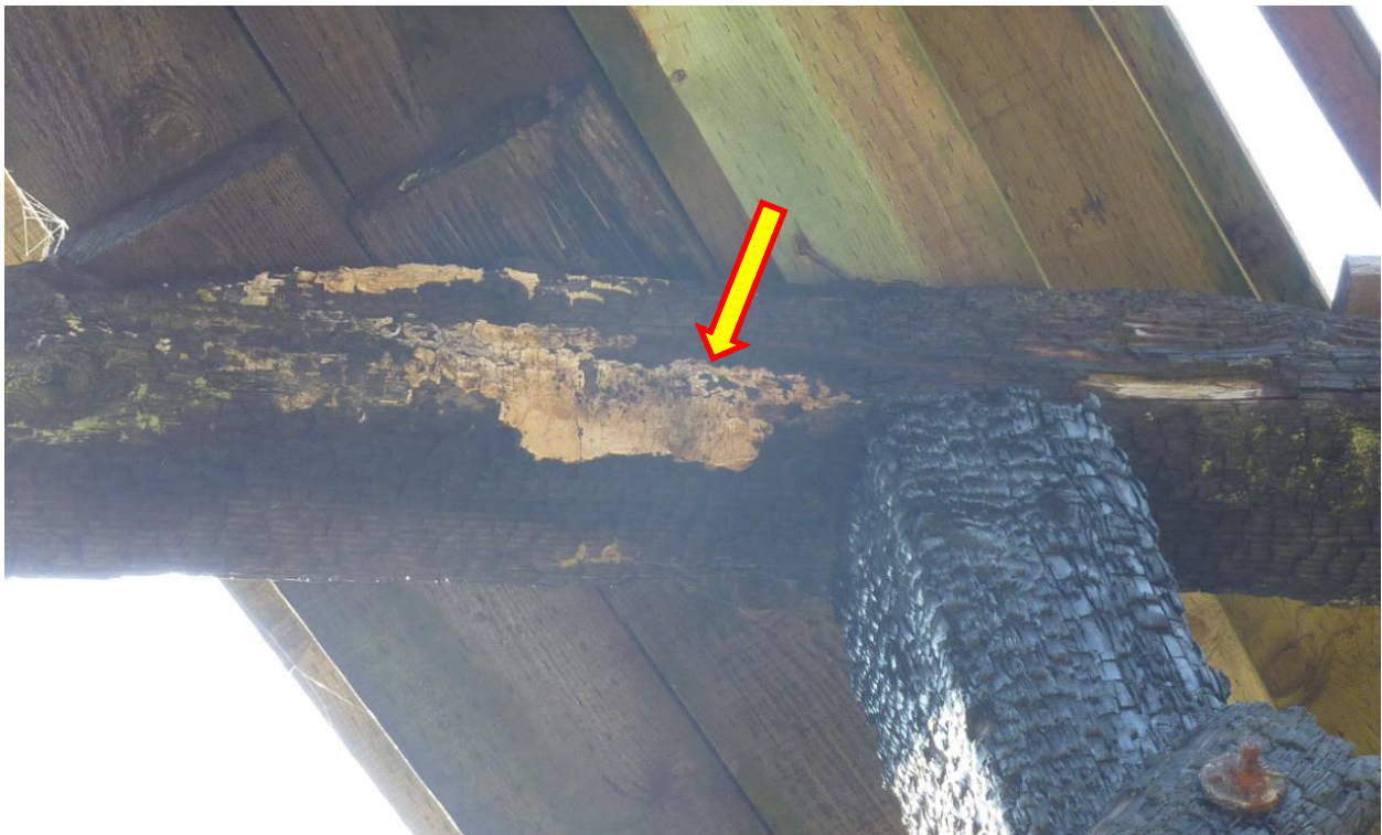
Figure 4. Organic growth on underside of 12x12 timber beam supporting temporary plank decking above.
