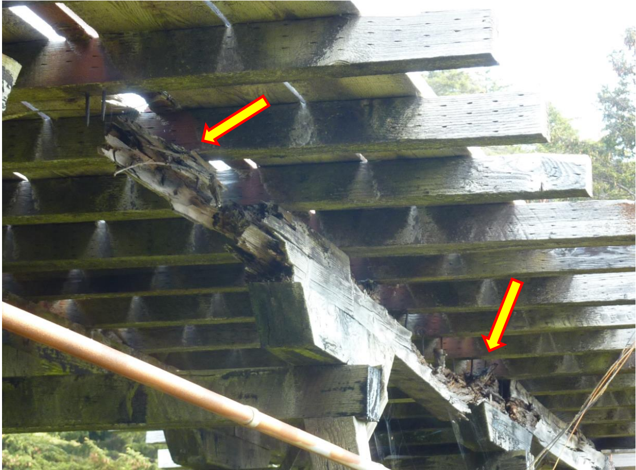
Figure 2. Joists supporting the tramway deck have lost integrity due to wood decay.
